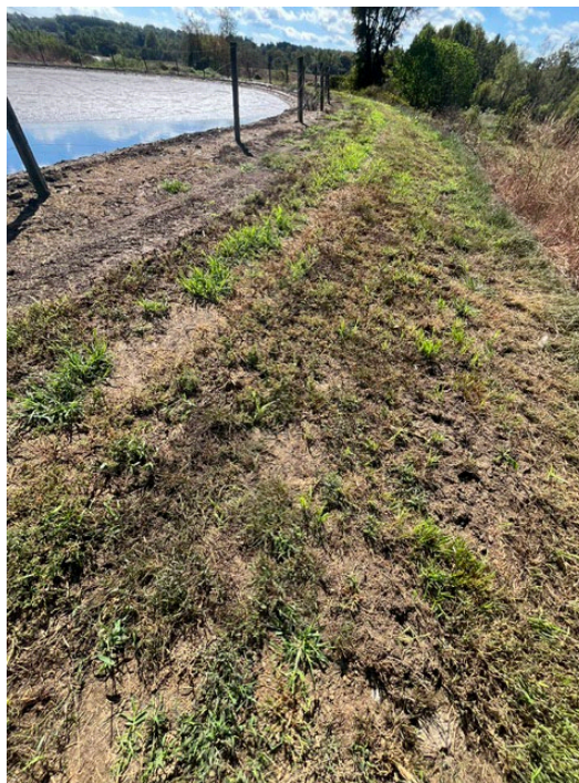
Manure pit # 3 – west side of the manure pit, which is the likely path the overflow took.
