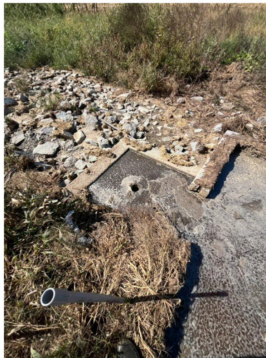
Collection basin showing a clogged pipe which leads To the holding tank and is pumped into manure pit # 3
