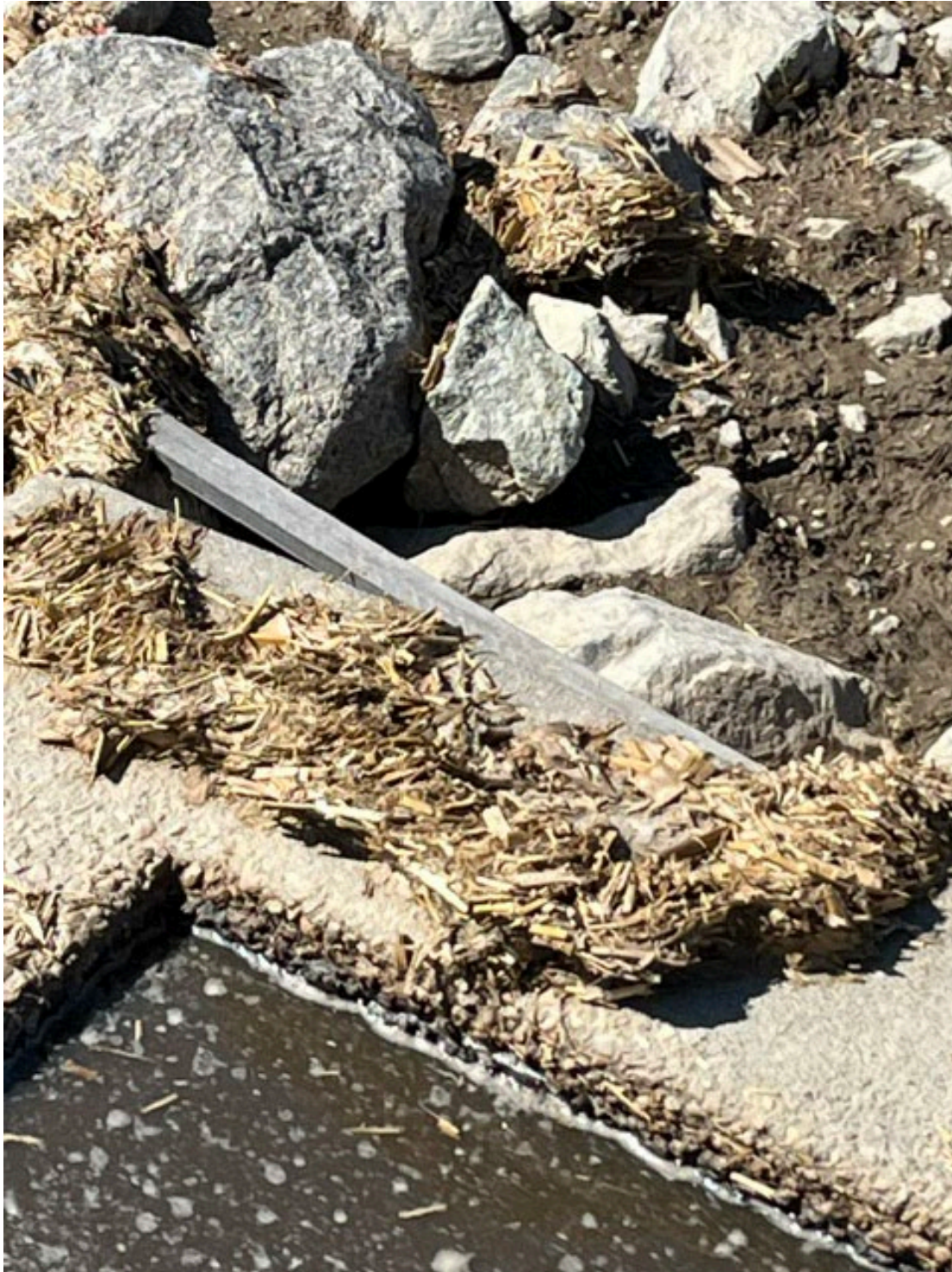
Top right corner of the leachate catch basin which had recently spilled over. On top of the basin wall is Silage which is a known pollutant.
